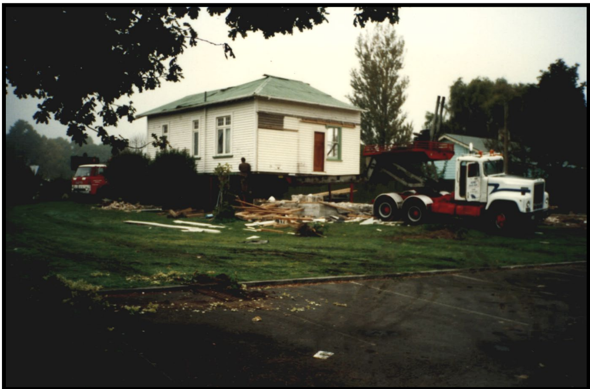
Figure 17: Houses at 921 Heaphy Terrace being removed to start construction of Hamilton Masjid, May 1997.
